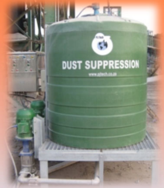
TANK WITH PUMPS
